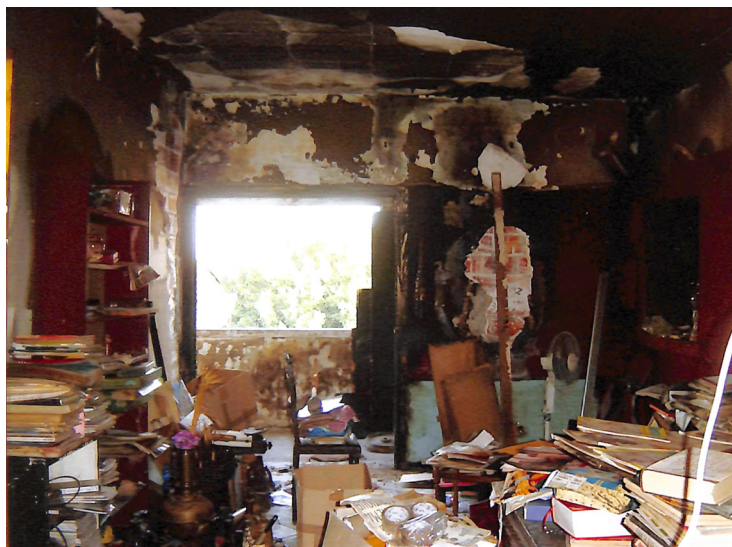
Figure 2: The Bouanani apartment after the fire in 2006, ©Touda Bouanani
